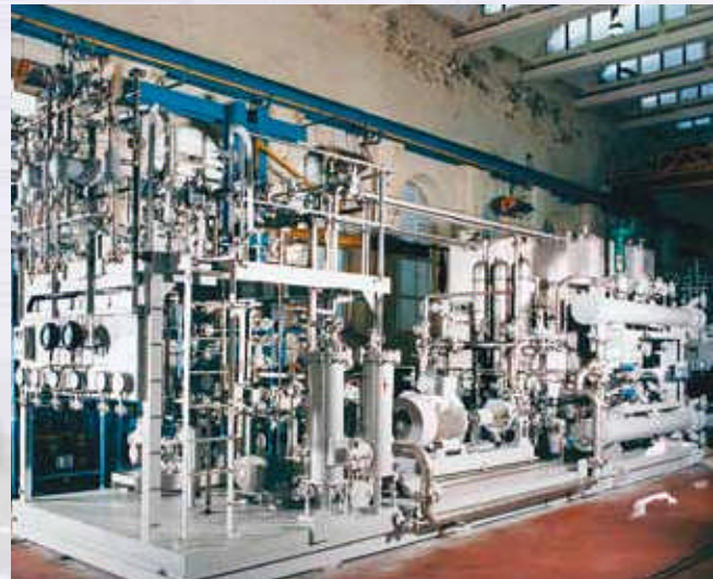
Compressed air cooling
